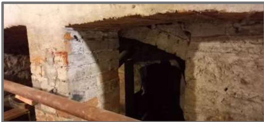
Remains of a fireplace- suggests this is part of the Victorian coal-fired boiler system.
